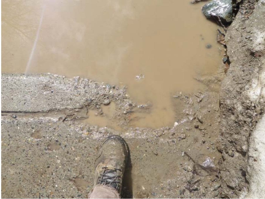
Left ballast wall damage
